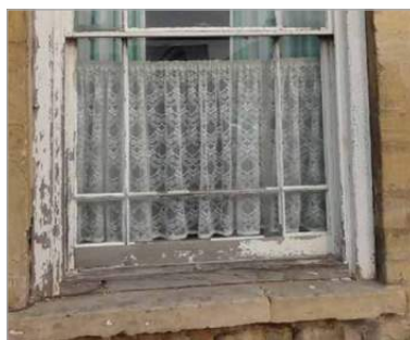
Lost putty around glazing and a lack of repainting can lead to air leakages
