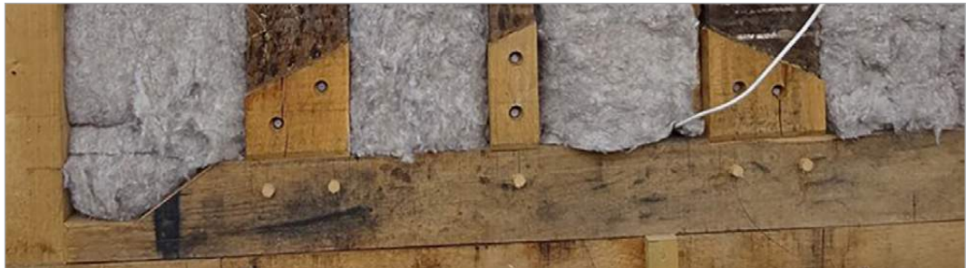
Insulation between existing and historic timbers would not damage the overall character of the property
