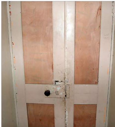
Insulating panels that integrate with the original design and repairs to cracks do not harm the historic character of the door
