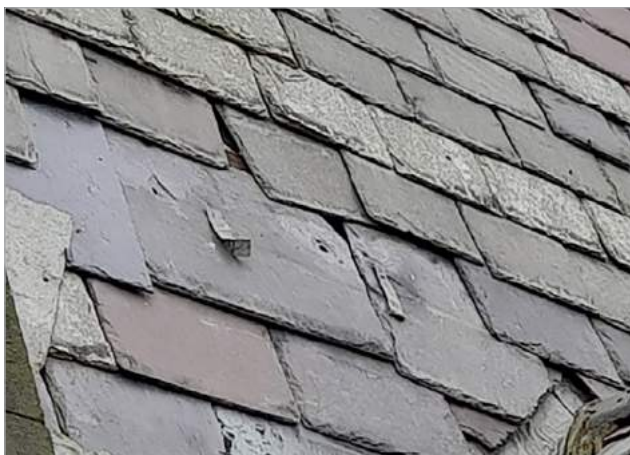
Missing or shifted tiles can allow water ingress causing damp inside the home
