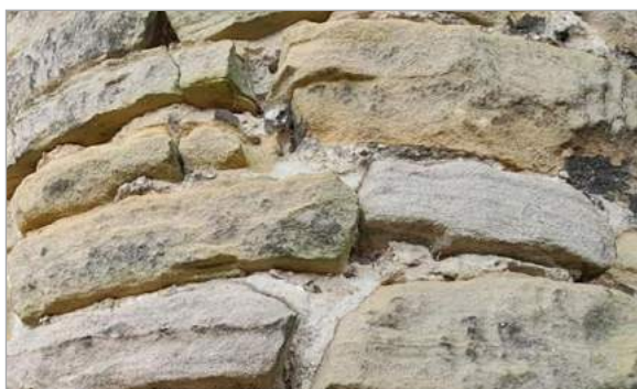
Missing mortar can lead to structural issues and water ingress if not maintained.
