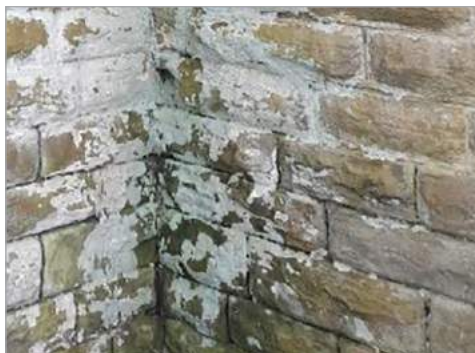
Moss and lichen build-up leads to consistently damp masonry
