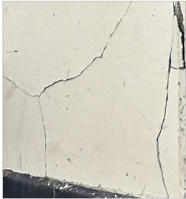
Cracks in render must be patched appropriately to prevent water ingress
