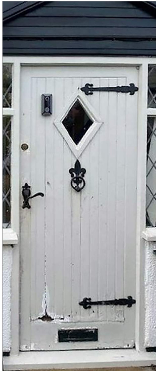
Repairing cracks or splits in door will also help reduce heat loss
